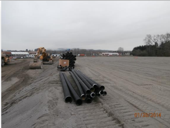
Utility piping and south parking lot
