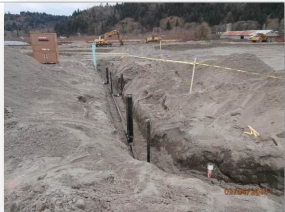
Sanitary sewer lines under building near service entry
