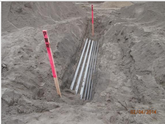
Underground electrical conduits along south edge of building
